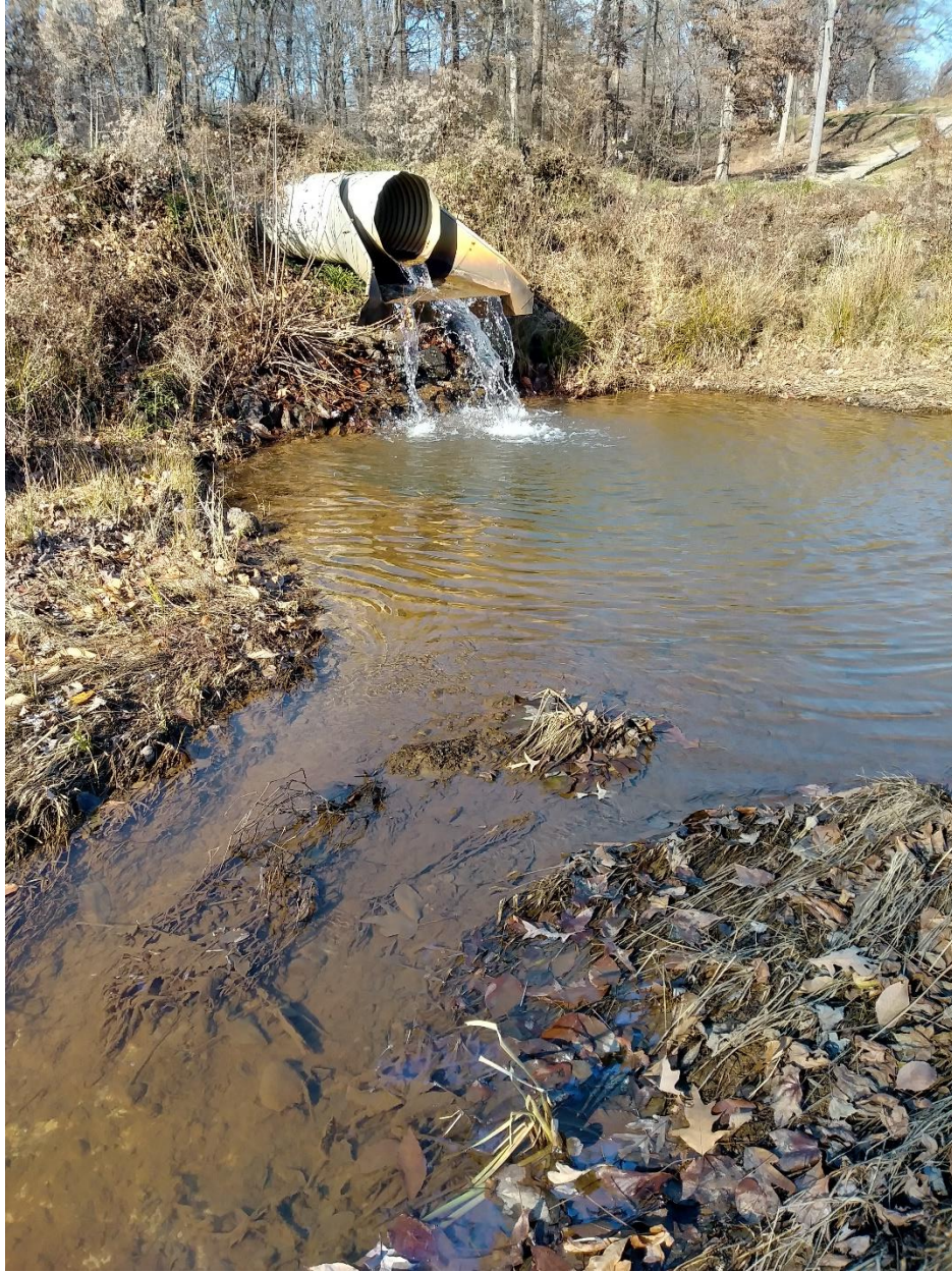
Site 4: 38°59'39.2"N 76°57'09.8"W. Water from site 3 pouring out of a rusty metal culvert into a low-lying bowl. This depression floods during large precipitation events.
